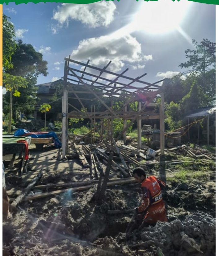
In Sorsogon, a resident digs out a mud-filled drainage canal in front of a house being built in place of one washed away by Kristine's floodwaters.
